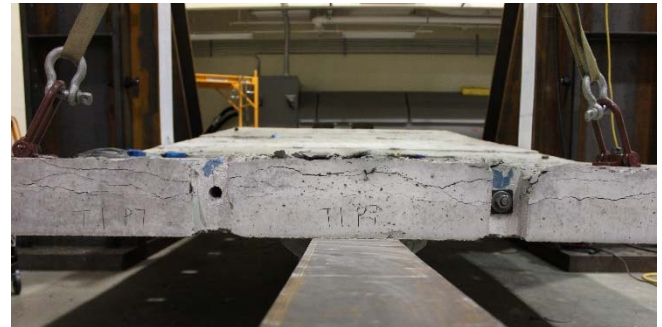
b) Concrete crushing at interior loading point (plastic hinge region)
