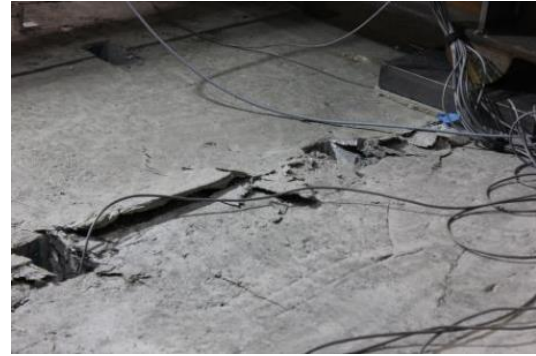
Fig. 11. Localized concrete crushing in specimen 2-m24-c1 at 190 mm deflection
