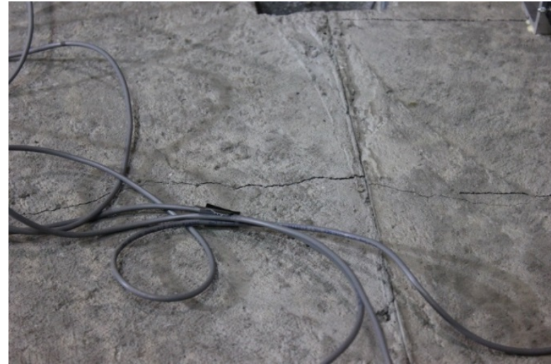
Longitudinal cracking (parallel to the steel beam)
