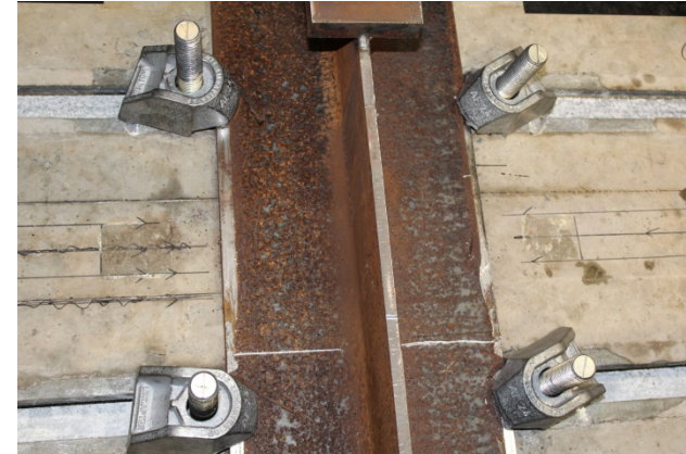
Abrasion on steel flanges
